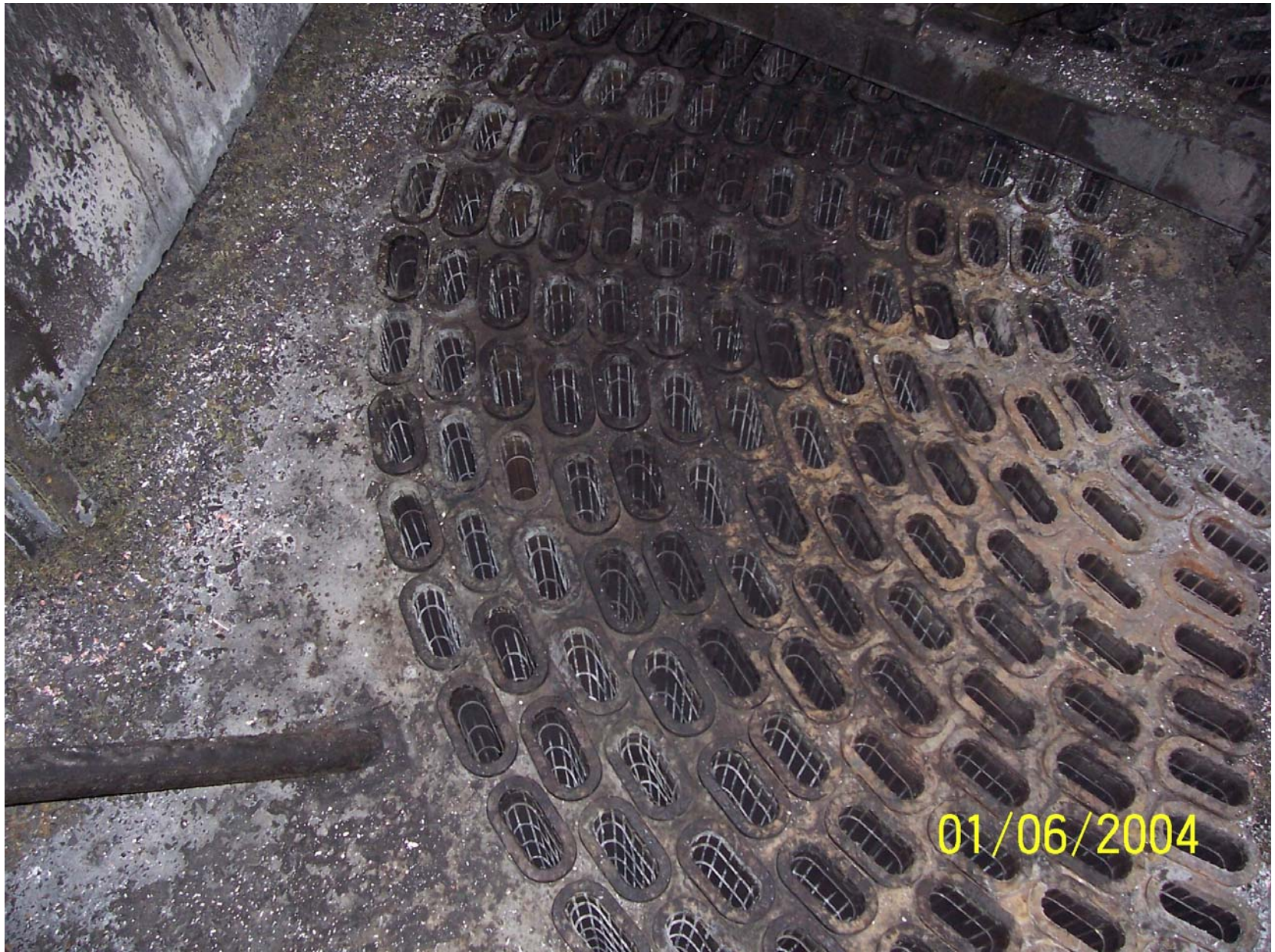
E. C. Gaston COHPAC Baghouse Tubesheet
