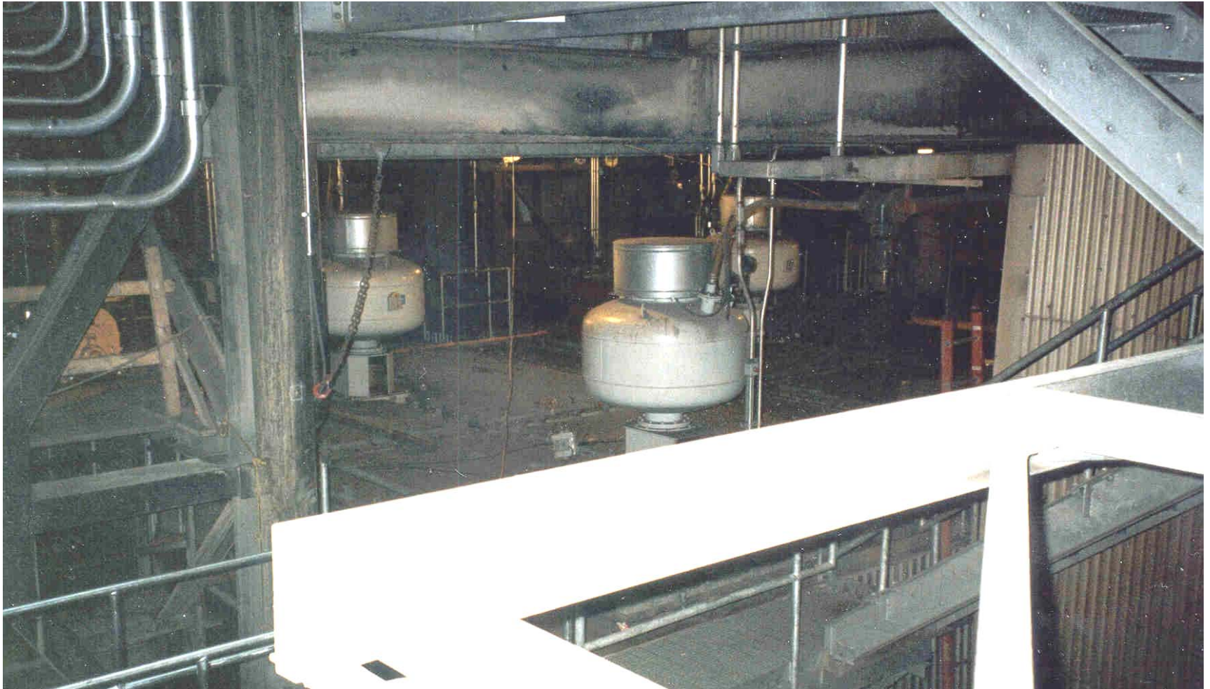
E. C. Gaston Unit 3 COHPAC Baghouse Casing and Pulse Reservoirs
